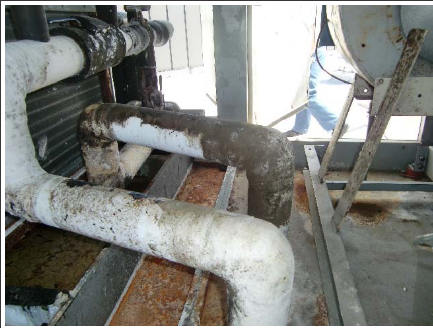
Air Handling Unit in Need of Remediation
